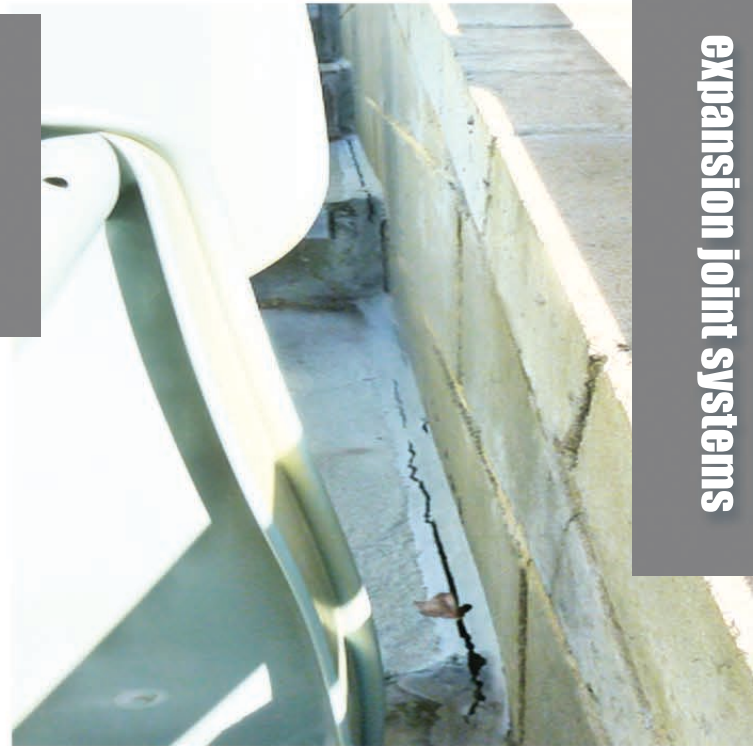
Stadium expansion joints are notorious for failure. This is due to the irregular 'round' shape of the Stadium bowl.
